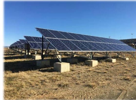
281 kW solar PV installation serving Moshoeshoe I International Airport
