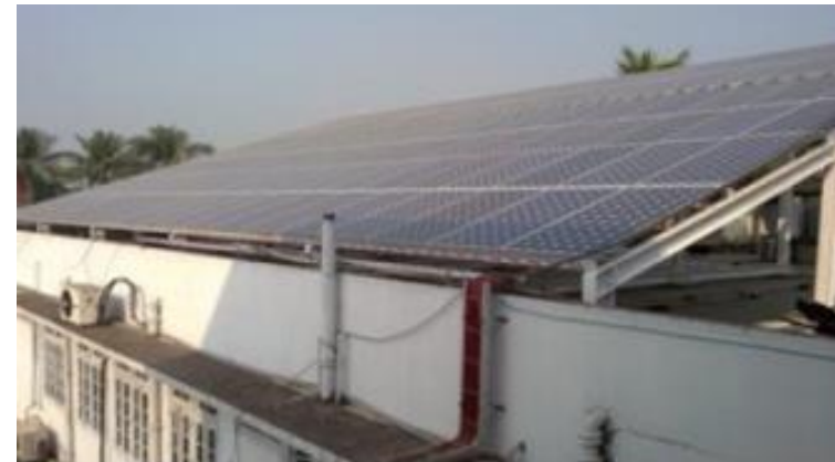
20.16 kWp PV Solar Power System at Honorable Prime Minister's Office, Dhaka
