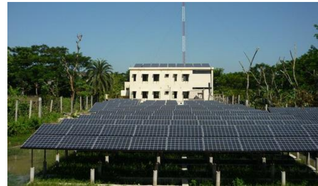
100 kW solar PV minigrid on Sandwip Island Source: Prokaushali Sangsad Ltd.
