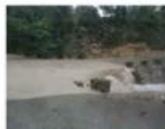
Roche a Bateau. Flooded road Credit: Cote Sud Initiative
