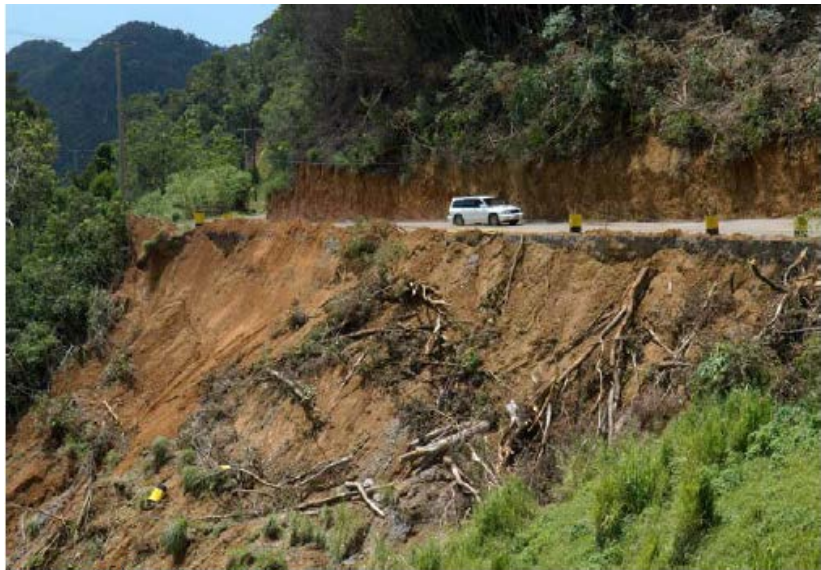
Major landslide on Imperial Highway
