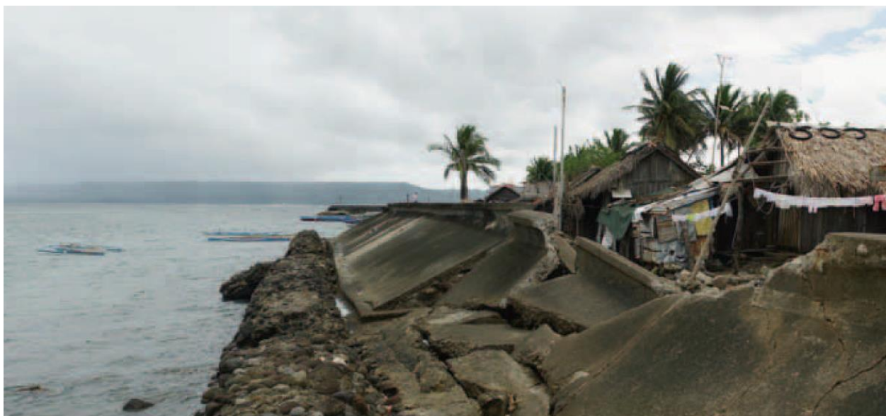
Figure 13: Damaged seawall, Bacon District, Sorsogon
