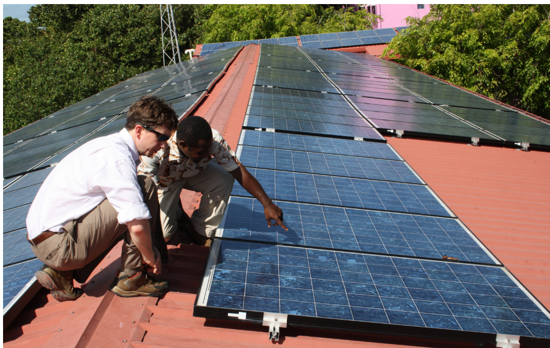
Solar PV System Installations, Muhyiddeen School, Villi-Male, Maldives. Photo: Renata Lukasiewicz/CIF AU
