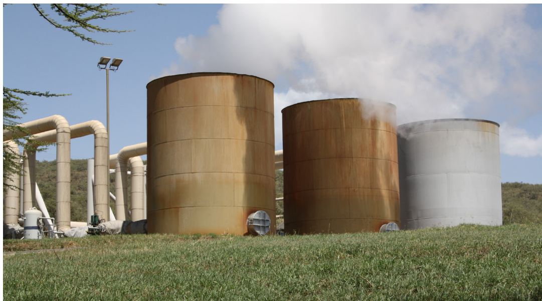
Olkaria Geothermal Plant, Kenya. Photo: Nasser Brahim/CIF AU
