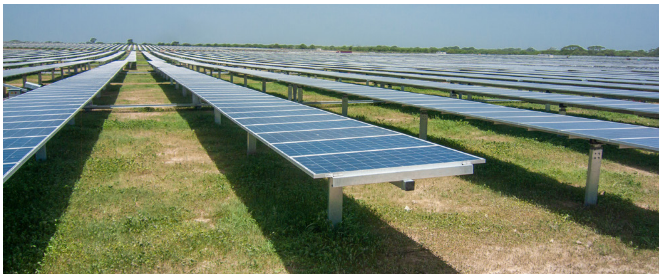
A solar power plant in Honduras
