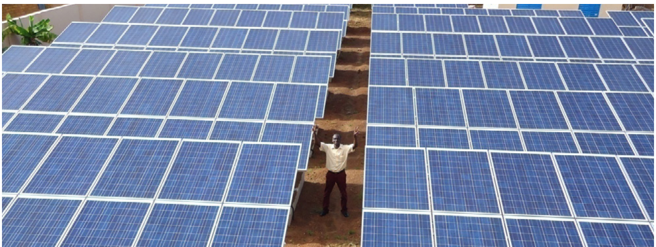
Solar facility in Kolondiéba, Mali
