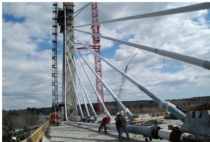
Figure 8: HDPE sheathing was used in combination with the cradles to achieve an air tight nitrogen filled seal around each stay.
