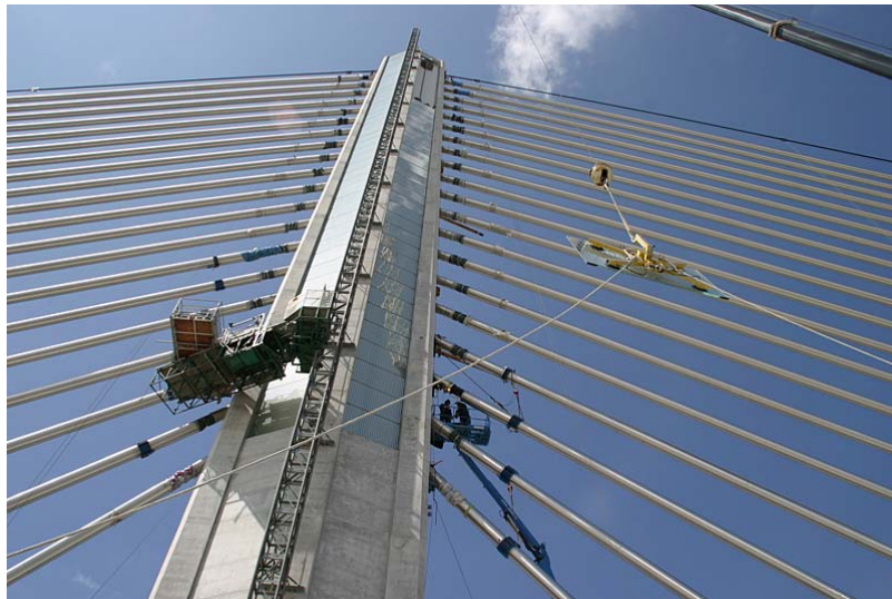
Figure 5: Glass being installed on the concave faces of the 23ft wide single pylon of the Veteran's City Skywalk Bridge in Ohio. The slender design was made possible due to the use of the cradle.
