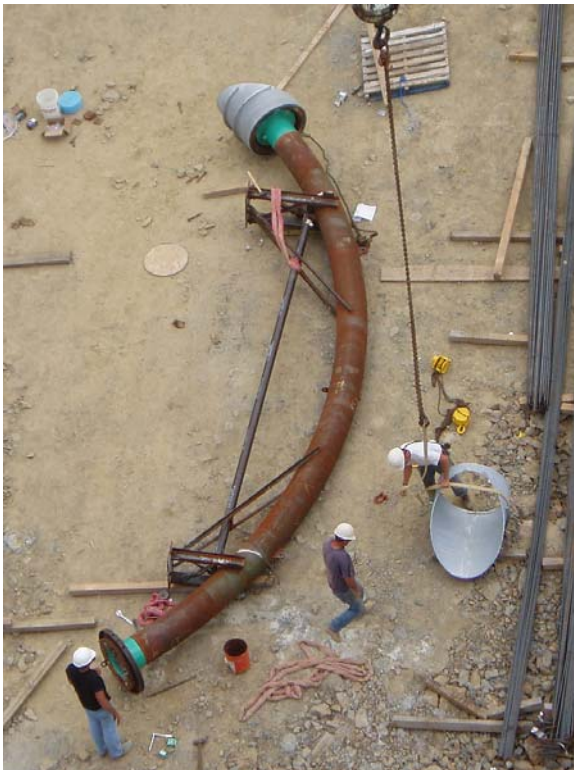
Figure 4: The cradle assembly is completed on site; it is fitted into a steel framework, and then lifted into position at each stay level.
