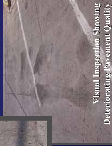
Asphalt and Aggregate Separation
