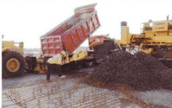
Figure 3- PMC receiving concrete and placing it front of the slip form paver
