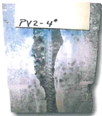
Cross section of blockwall cell illustrating improper vibration technique
