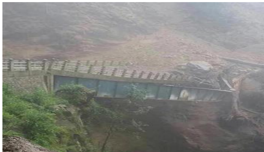
Figure 5. Dokumlung bridge damage by landslide
